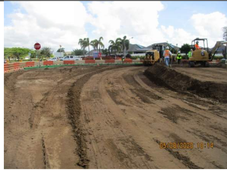
Roadway excavation from Sta. 49+00 on Maui Lani Parkway to Sta. 10+60 on Kamehameha Avenue.
