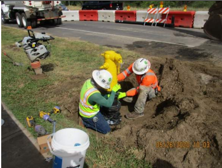
Install new fire hydrant with a 12-inch extension at Sta. 8+60 on Kamehameha Avenue.
