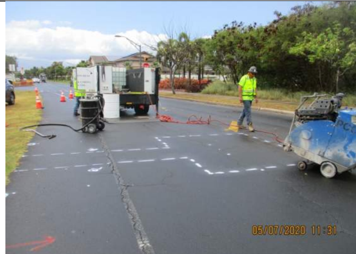
Saw cut layout for the new fire hydrant at Sta. 52+51 on Maui Lani Parkway.
